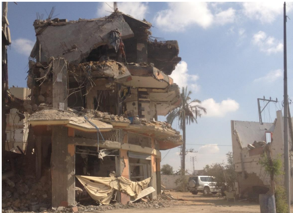
Many houses are completely destroyed or seriously damaged in the Gaza Strip. © SDC
